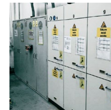
HAZARDOUS SUBSTANCES CABINET WITH TECHNICAL VENTILATION
