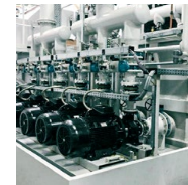
SECONDARY PROTECTION FOR COOLING LUBRICANT: CENTRAL UNITS
