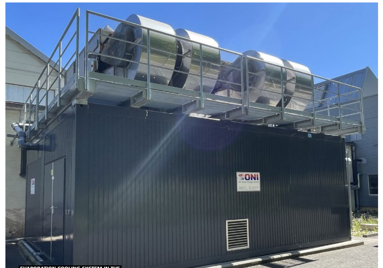
EVAPORATION COOLING SYSTEM IN THE INDUSTRIAL COMPONENTS DIVISION
