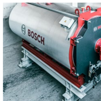
NEWLY INSTALLED BOILER IN BOILER HOUSE
