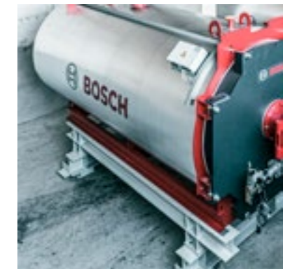
NEWLY INSTALLED BOILERS IN THE BOILER HOUSE
