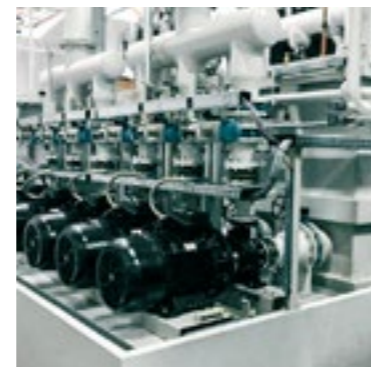
SECONDARY PROTECTION FOR COOLING LUBRICANT: CENTRAL UNITS
